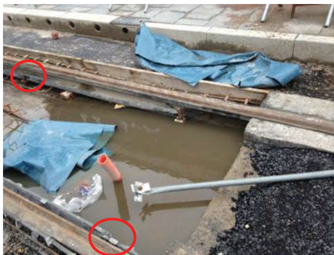
Figure 12. Missing insulation at clips and missing rail boot overlap.
