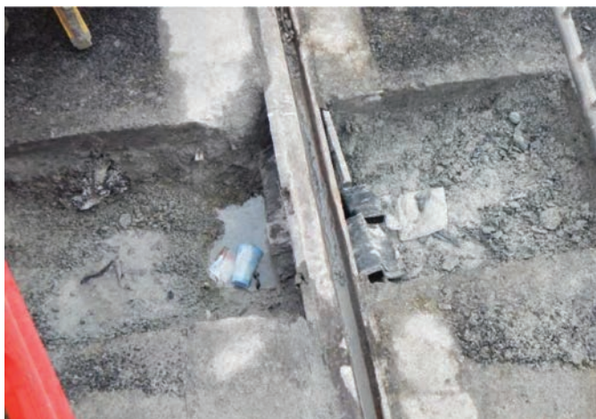
Figure 11. Broken rubber boot on the rail requiring excavation.
