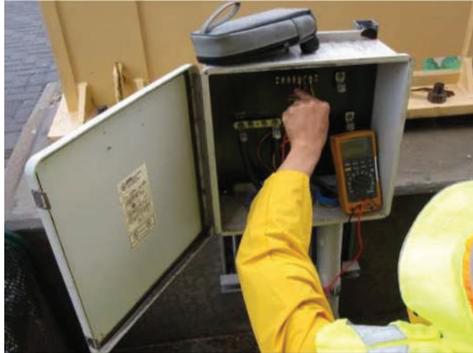
Figure 17. Example 1: utility testing station.
