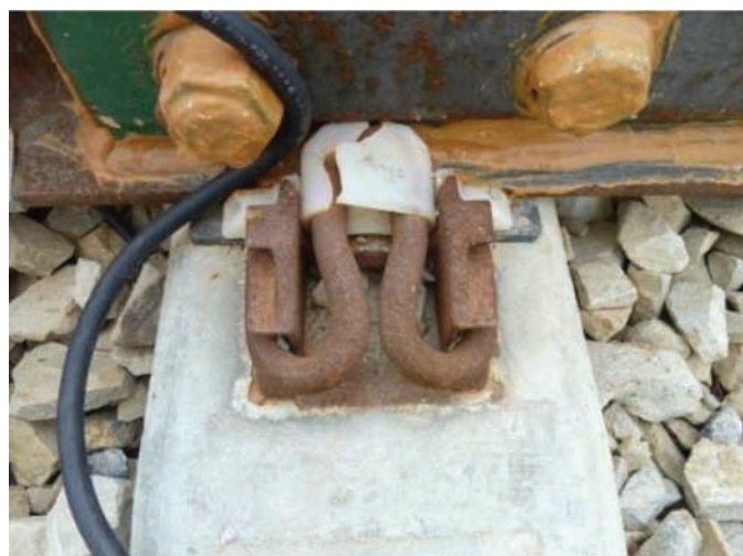
Figure 10. Cracked insulation cap on the fastener clip.
