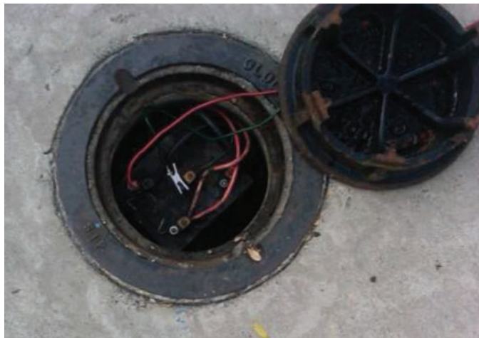
Figure 18. Example 2: utility testing station.
