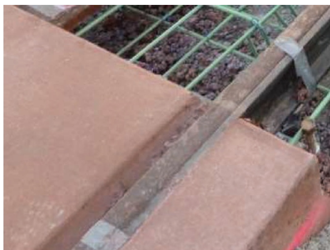
Figure 14. Tee rail with rail boot and concrete groove.
