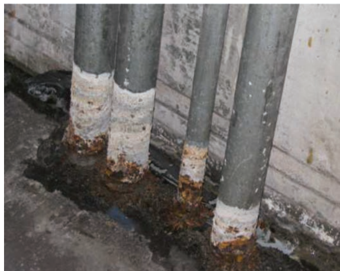
Figure 21. Corrosion of pipes at station facility.
